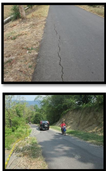
Picture 1.5 soil cracks and landslides on the Sidamukti road section
