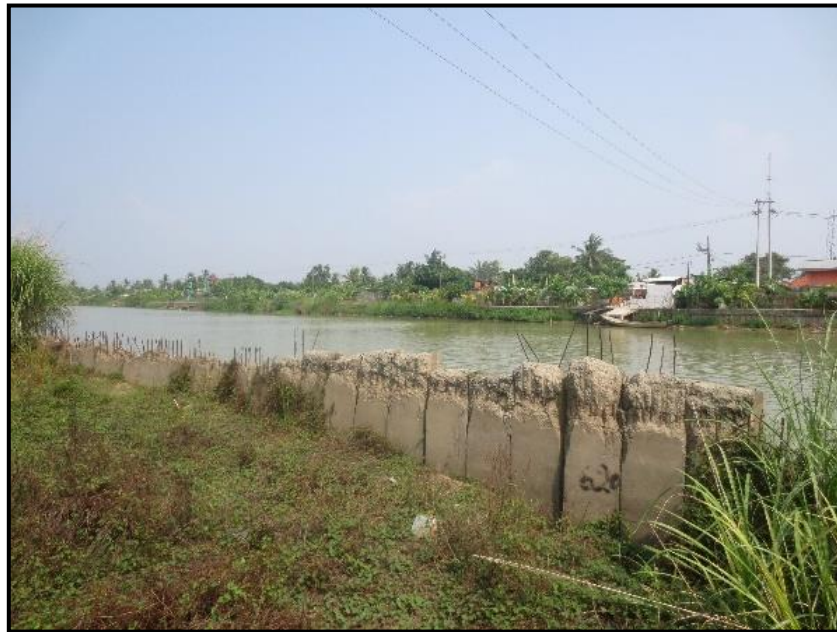
Figure 4. One of embankment burst point due to heavy rain fall in 2017
